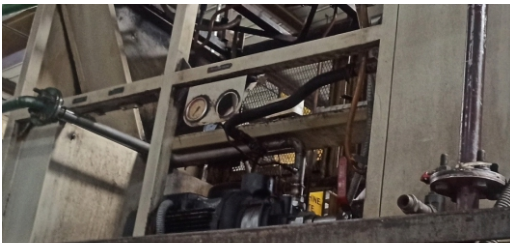
Chiller Guards Were Missing Both Side
