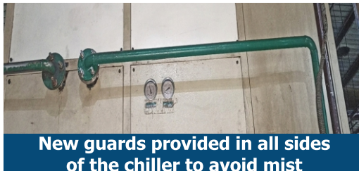
New guards provided in all sides of the chiller to avoid mist deposition in the copper tubes.
